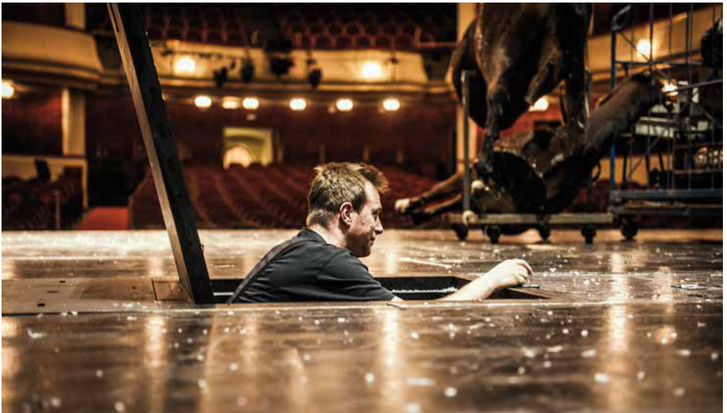
14:08 Open-heart surgery: renovation work on the stage means performing a complex operation on the theater’s most sensitive part.
